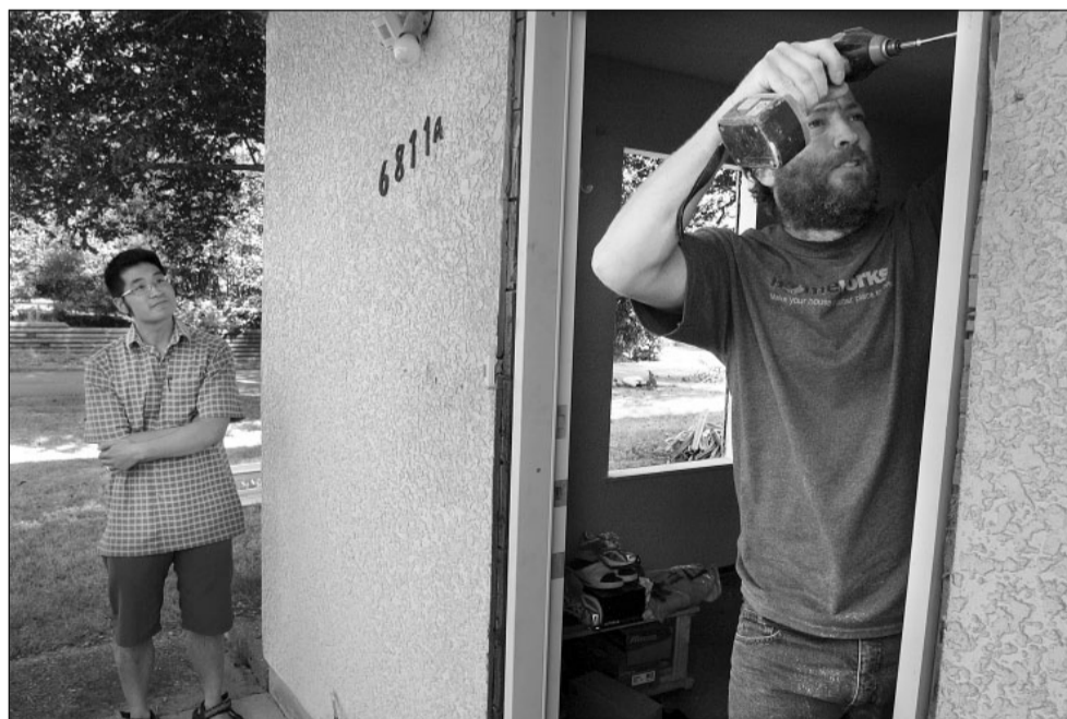
Jason Lee keeps a close eye on the proceedings as a crew of workers replaces doors, windows, insulation and furnaces in his Burnaby duplex to make it more energy efficient.
